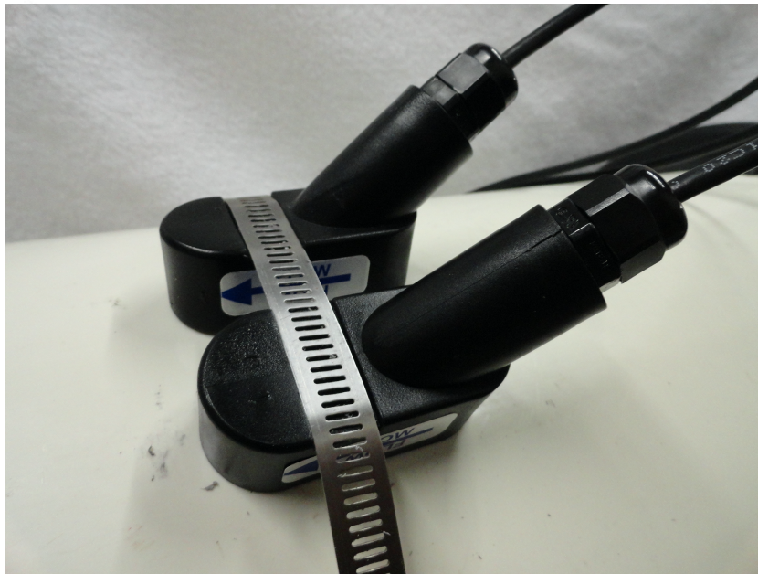
Figure 2-5. Clamp-on transducers secured with a bungee and chain
