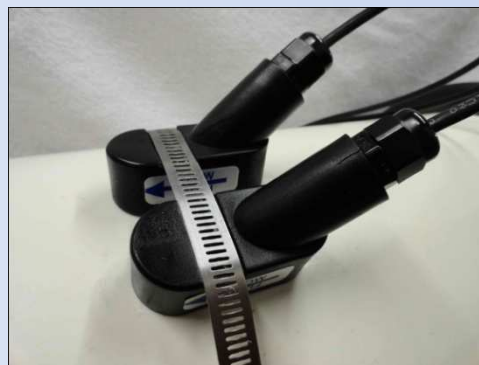
Figure 3. Clamp-on transducers secured with a SS ½" gear clamp band
